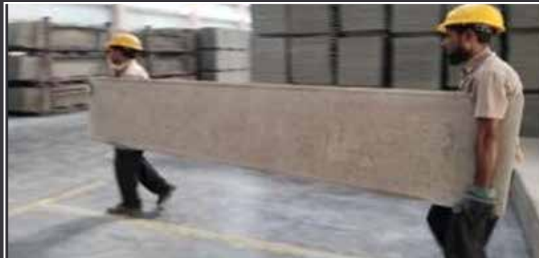
Lift and carry the Vpanels vertically as far as possible for ease of shifting and convenience.
